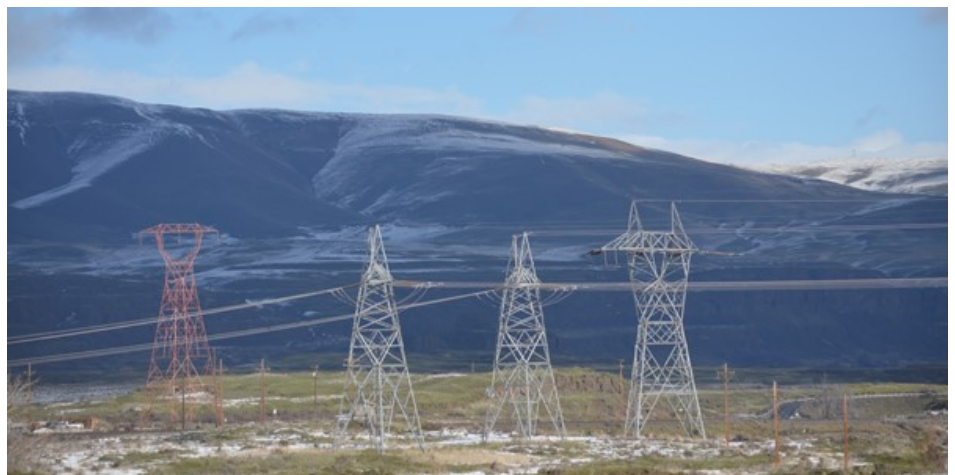
BPA transmission line in Klickitat County, Wash. | © RTO Insider
